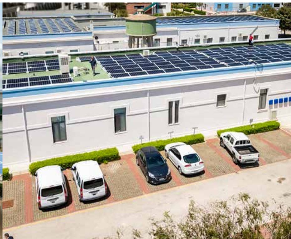
PV Panels at UNGSC in Brindisi. UN Photo/Luca Nestola.
