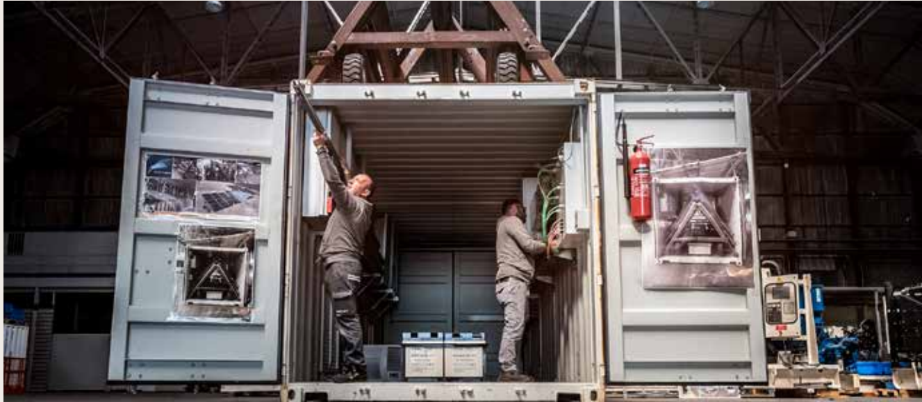
Smart containerized photovoltaic (PV) plant, first version. UN Photo/Luca Nestola.
