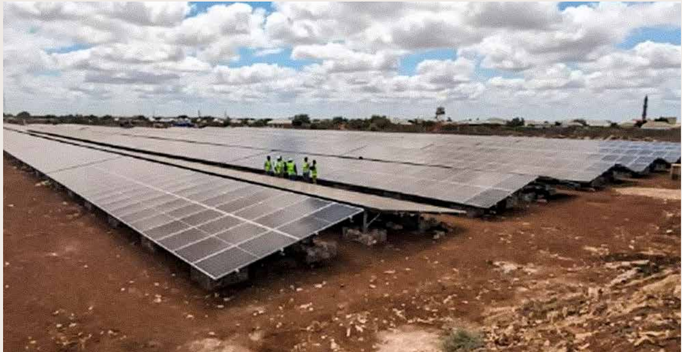
Baidoa solar photovoltaic power plant. Source: Kube Energy.
